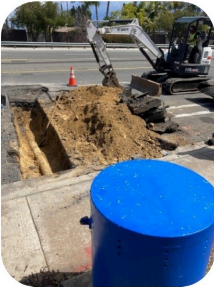
Photo: Air release valve (blue can) and associated pipeline and appurtenance replacement construction
